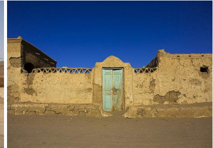
Figure (39) Cob wall plaster (zibala) easily washed away by rainwater and removed by hot tropical sunrays and storm
