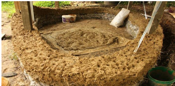
Figure (31) Mixture of soil, water and hay or chopped straw directly apply in walls, as in the cob method or madamik
