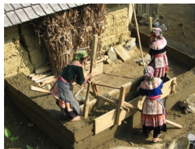
Figure (22) The two planks then raised up and a second course of rammed earth repeated
