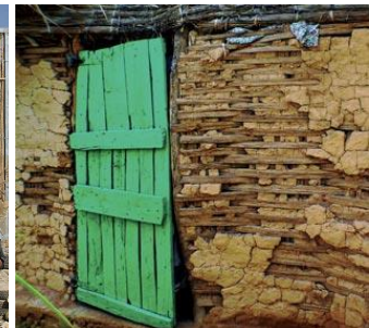
Figure (30) A wattle and daub wall washed away by rainwater
